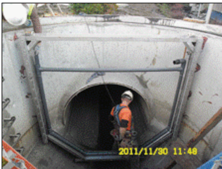
FIGURE 12.10 Polymer addition point at the Columbia Boulevard facility.
