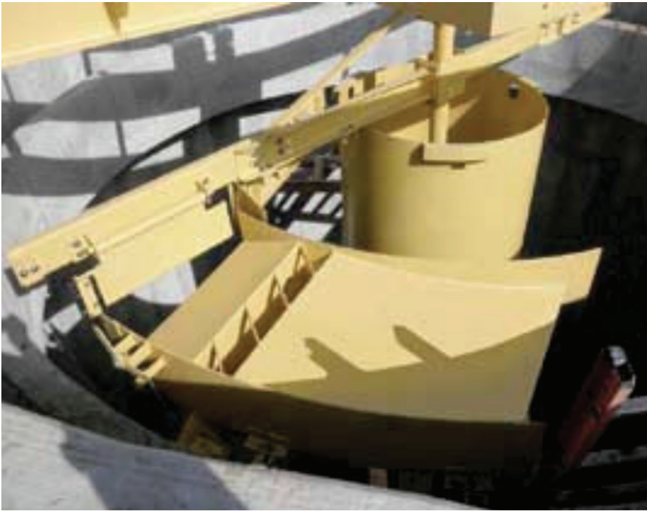
FIGURE 12.2 Scum box and beach plate at a small primary clarifier (courtesy of Monroe Environmental, Monroe, Michigan).
