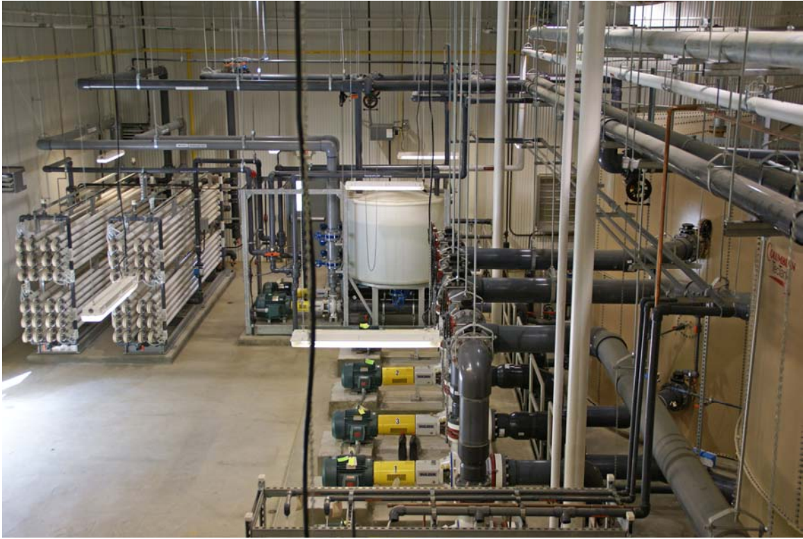
Figure 2. General View of the MBR Facility
