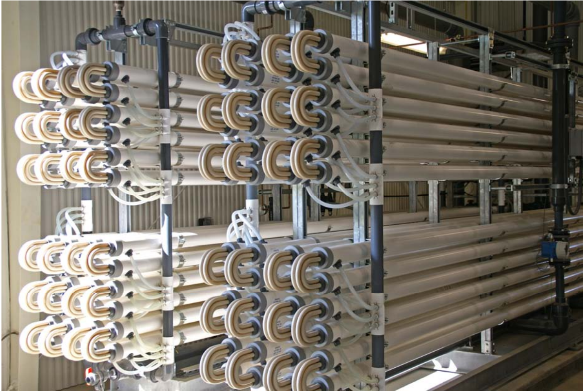
Figure 4. Battery of the UF Membranes
